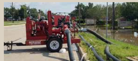
6" Pumps on FM 359 in front of District Office
