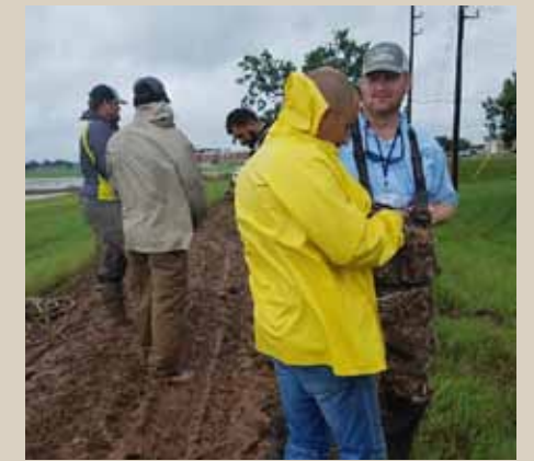
Director Howard & Director Yokubaitis Assisting with Coordination of Plug Installation at Plantation 4/5
