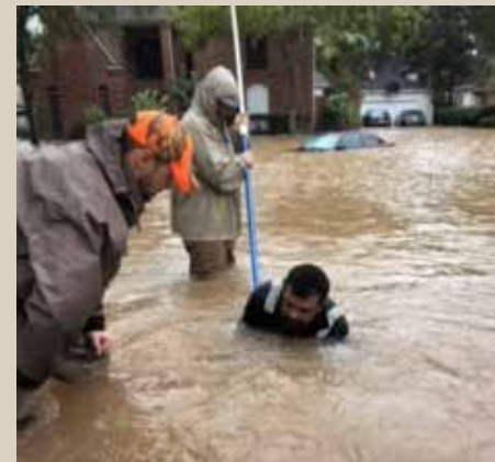
Director Yokubaitis & Dive Team Retrieving the Pull Cable from within the Manhole for Plug Installation
